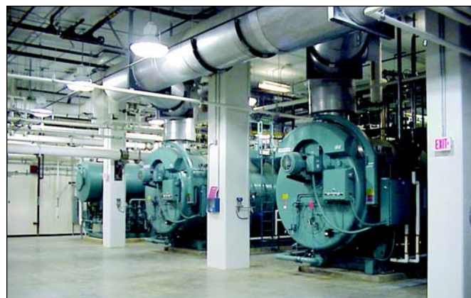
Plant steam boilers.
