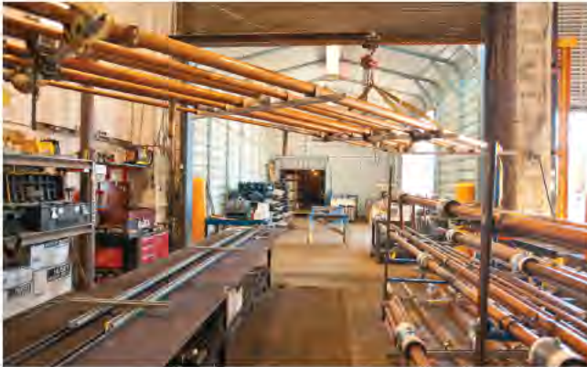
Figure 2. Prefabricated Racking of Services: prefabricated racks in the service corridor that includes all major utilities and services.
