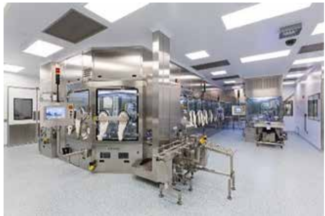
Figure 5: An open isolator enabling flow of nested tubs and vials through mouseholes. (Image courtesy of Catalent. © 2020 Catalent, Inc. All rights reserved.)
