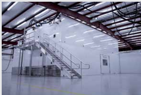
Figure 1: Prefabricated cleanroom unit (POD) with integrated air handling system in shell building
