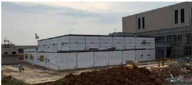
KUBio modular components are assembled to construct the GE Healthcare Life Sciences facility in Wuhan, China.
