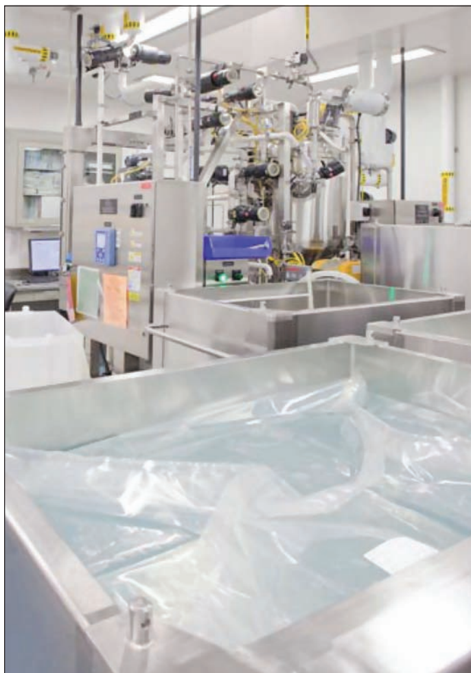
Mid volume buffer tote for UF operation.
