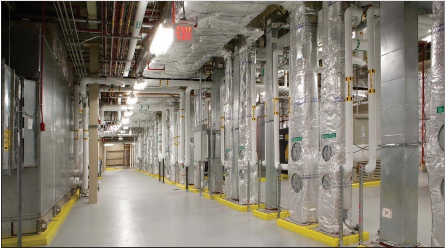
Stick-built mechanical mezzanine.
