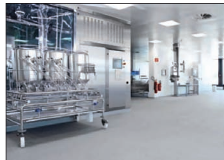
Novartis Vaccines and Diagnostics GmbH: segregation staging of equipment.
