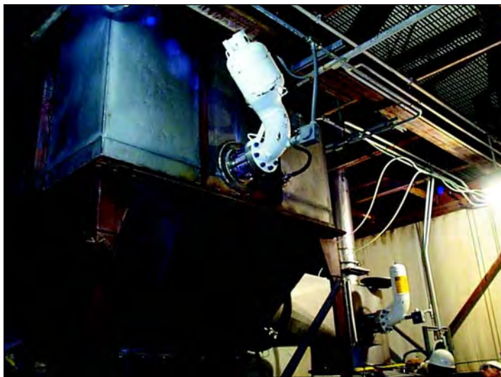
Dust collector with an explosion suppression system.
