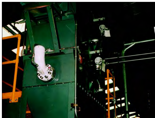
Figure 4. Explosion suppression system installed in a dust collector.
