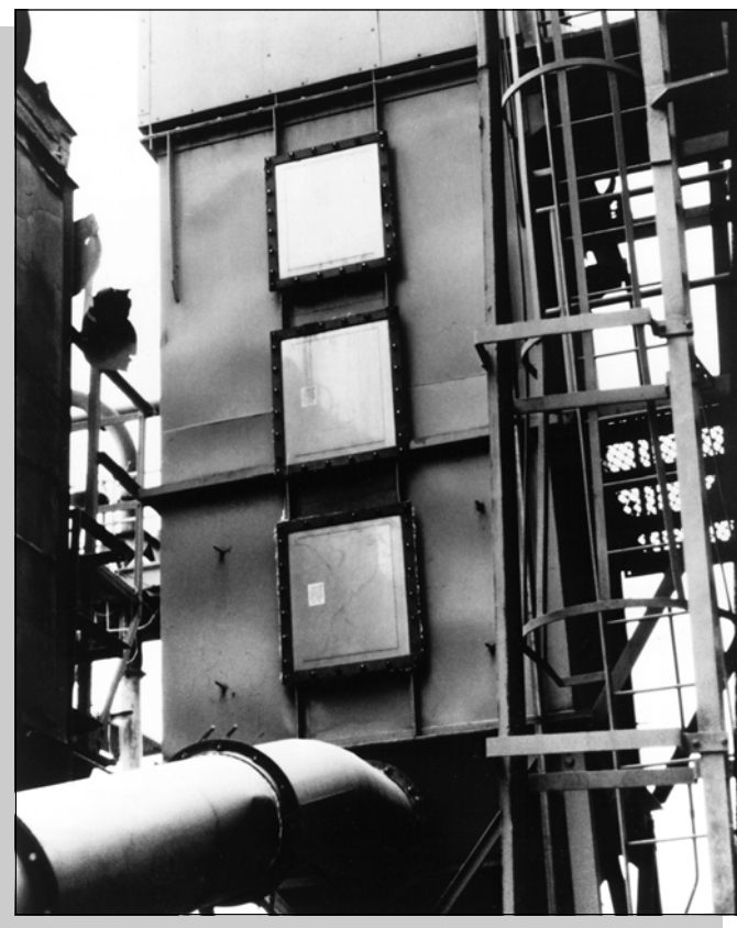
Figure 2. Typical explosion vents.
