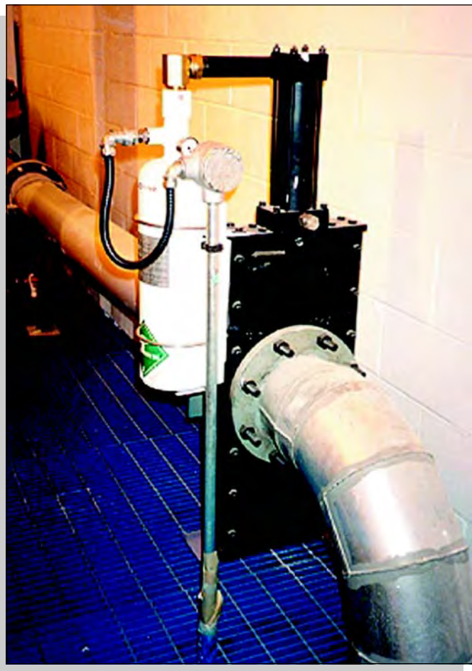
Figure 5. An explosion isolation valve.
