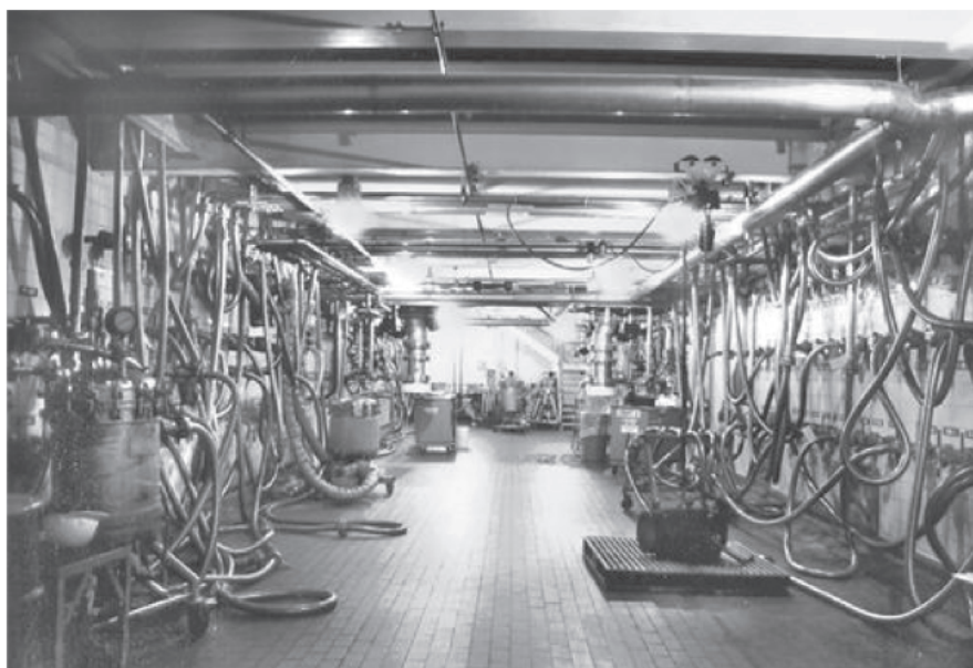
Figure 3. Main process transfer station in a 5 pool API plant set up for cleaning and process operations.
